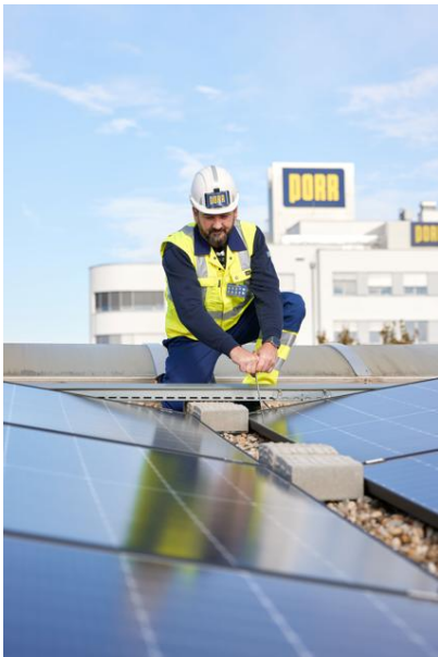
Expanding photovoltaic systems © Oberbramberger
