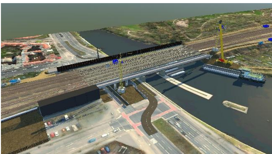
Work on heritage-protected buildings and beside existing railway tracks requires precise logistics and coordination © DB InfraGO AG
